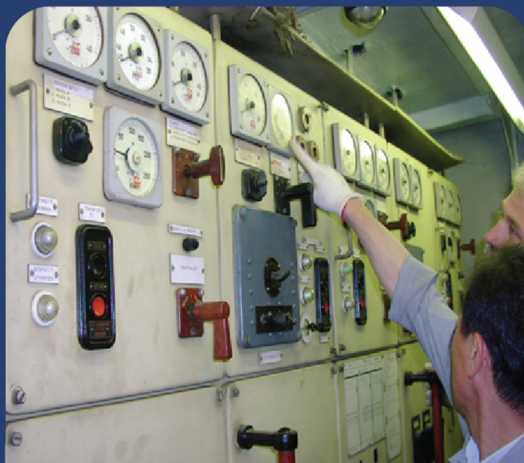
FAULT FINDING OF MAIN SWITCH BOARD
